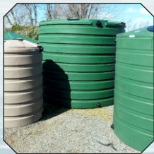
Water Tank Systems
